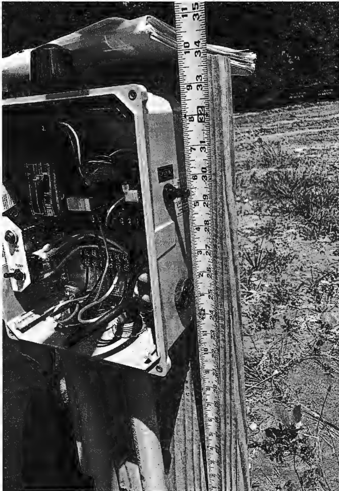
7/11/25 1st Inspection - Control panel is 24" to grade.
