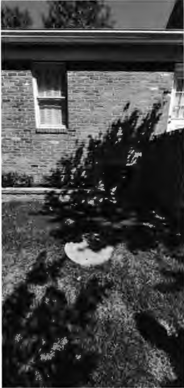
Septic Tank Clean-Out Cover
