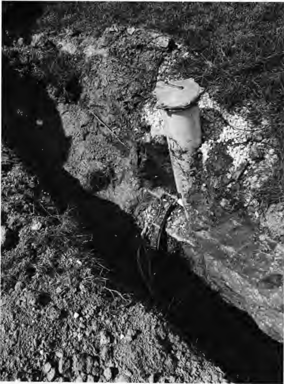
7/22/25 Existing well has been disconnected. Contractor tied in the new line to the existing line. (13)
