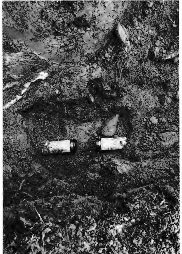
Septic tank front line capped
