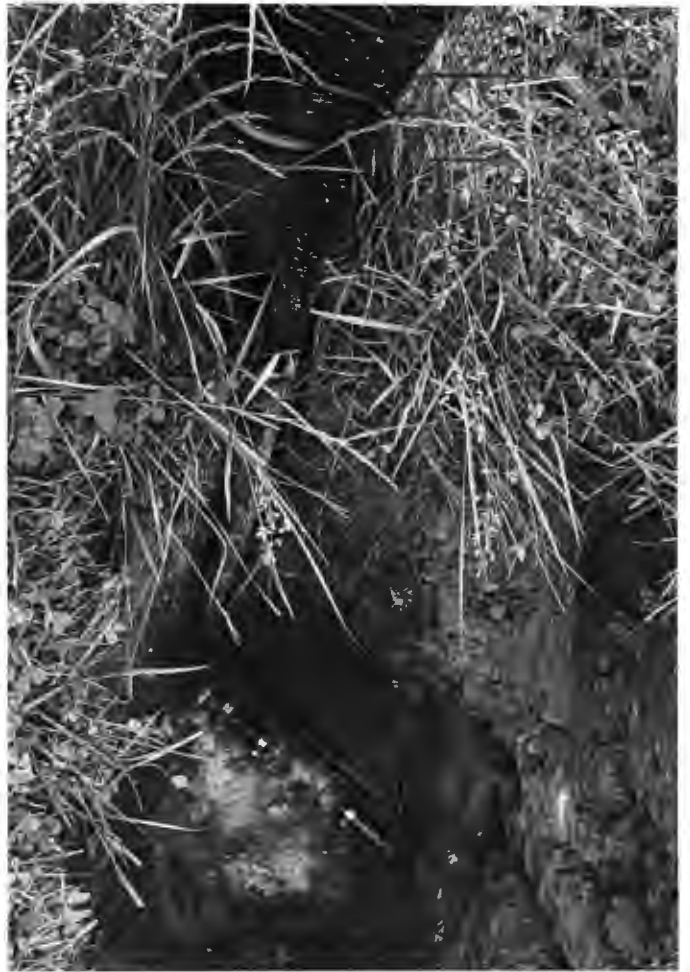
Well line capped
