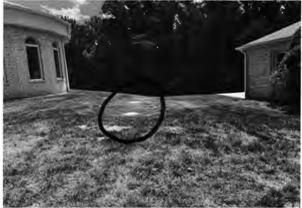
risers for septic tank installed w/out permit
