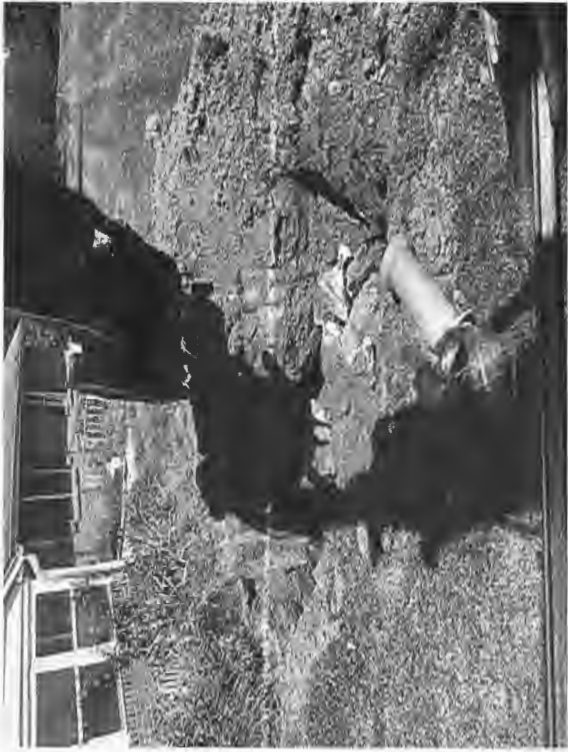
6485 SOUTH TROTTER ROAD EXISTING SEPTIC TANK COLLAPSE
