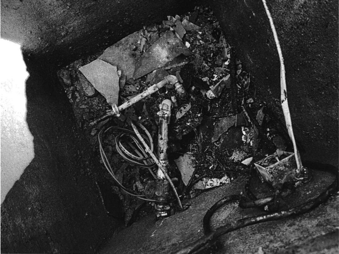
3663 Hipsley Mill Road – Pictures of ex. well capped off, ex. septic capped off. Completed on 9/1/2022
