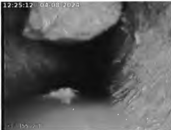
Junction with cast iron snakeline next to the driveway.
