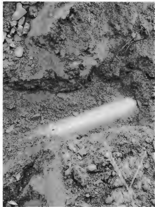
Picture above ↑ showing 4" electrical conduit coming from ex. Poly tank outlet.
