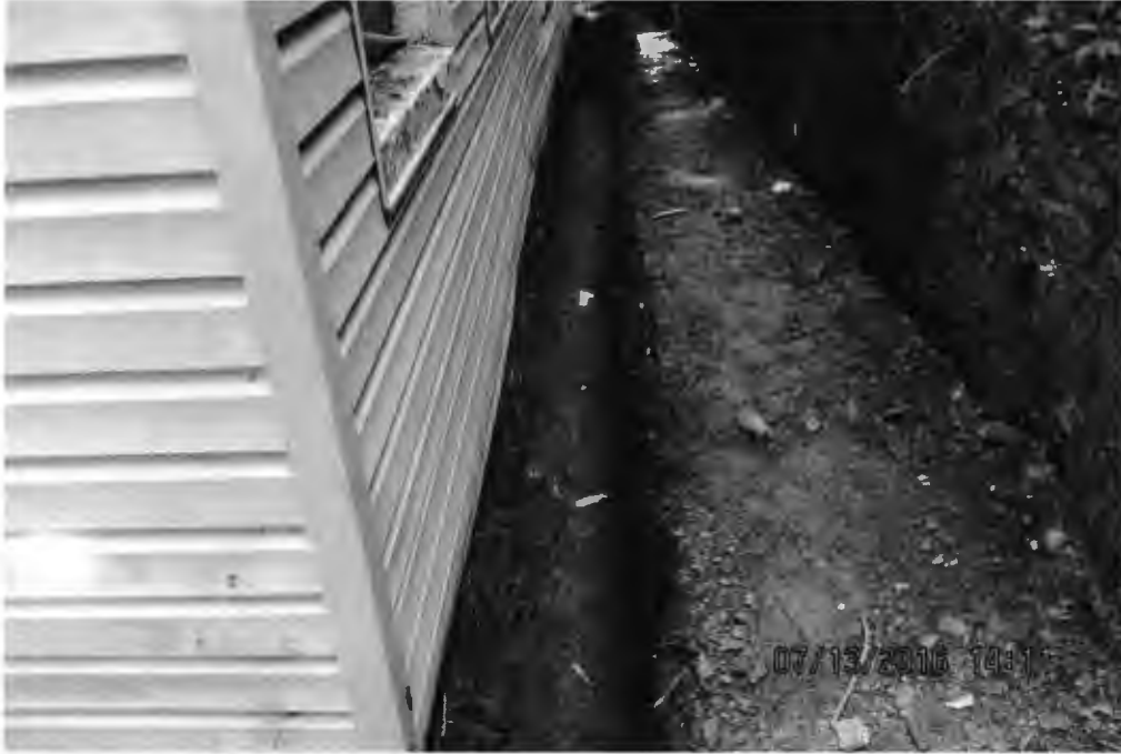
Trench dug on right left side of house for a footing or damp proofing. Owner could not explain how trench is to be used.
