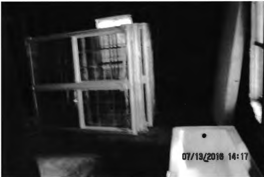
First floor- entire house is gutted
