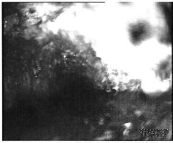
Water sitting in drain pipe to drywell
