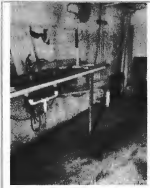
Picture 4: [Picture from original inspection] Showing the sink in the utility room behind the house. This sink must be rerouted to the septic system or be removed.
