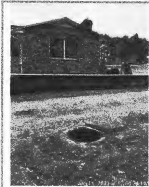
Picture 1: [Picture from original inspection] Showing the septic tank in relation to the house.
