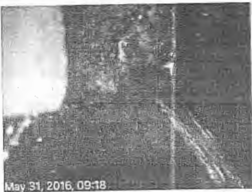
Picture 2: Water entering the septic tank through the front line. The septic tank is composed of cinder blocks.
