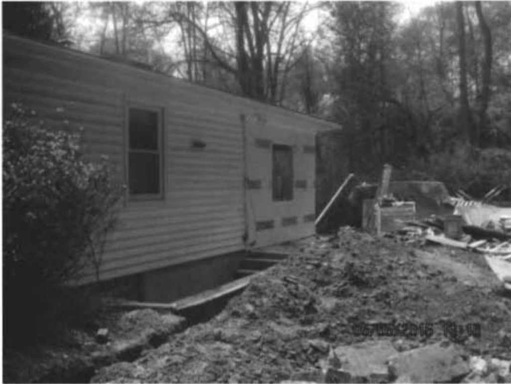
Trench with sewer line installed, running from rear of closed-in porch to septic tank.
