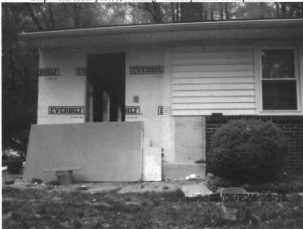
Covered porch on left side of house closed in for living space w/ plumbing.
