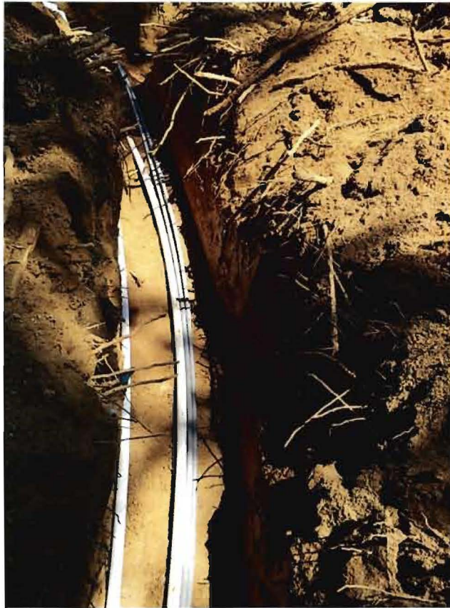
Electrical conduit, supply, and return lines
