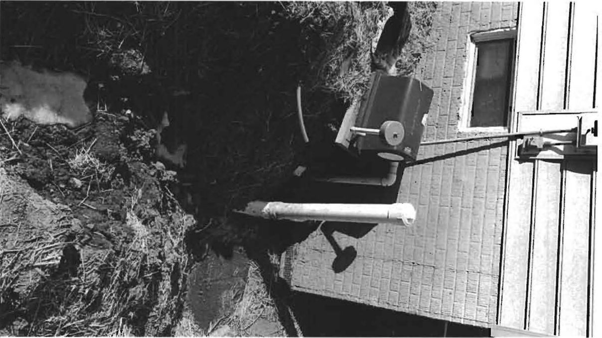
14528 Edgewoods Way Images of house connection from Jake at Fogle's
