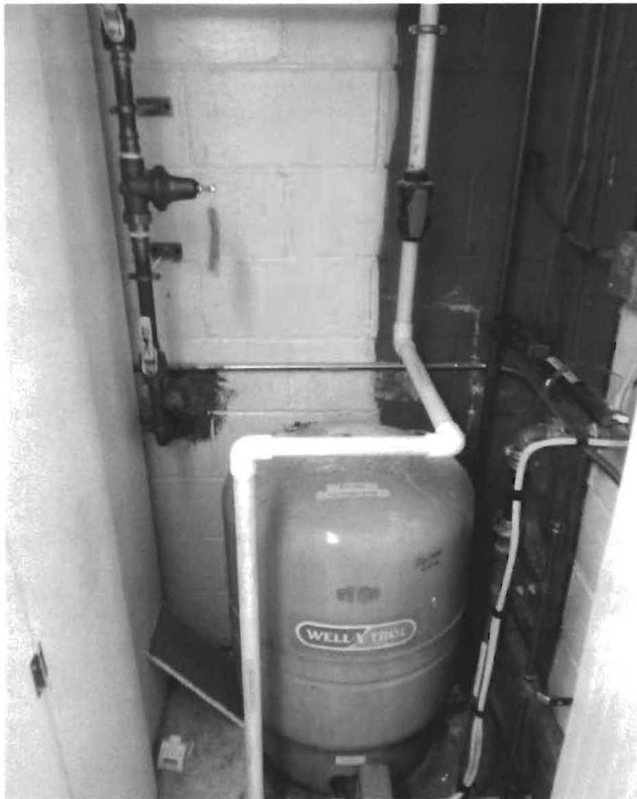
Well later lines are labeled as Non-Potable. (And only feed water to the hose bib located out front and the back yard spigot.)
